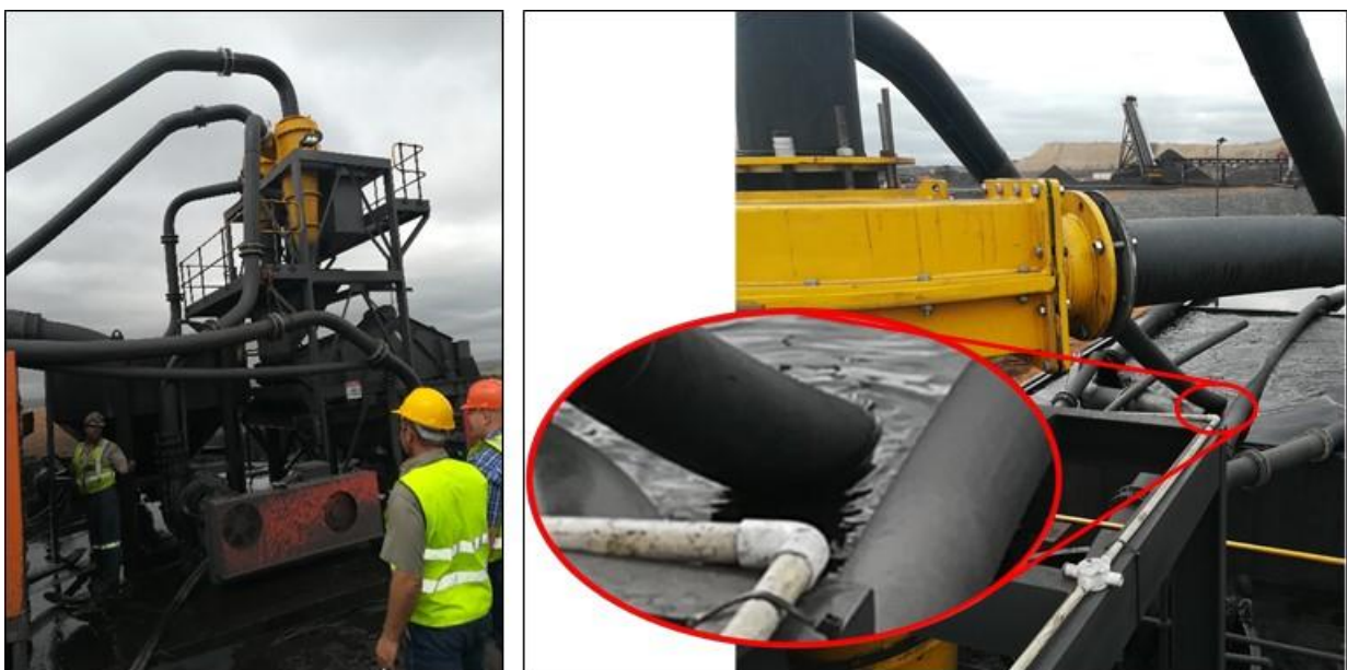
Figure 14: Siphoning created by inappropriate overflow installation.
