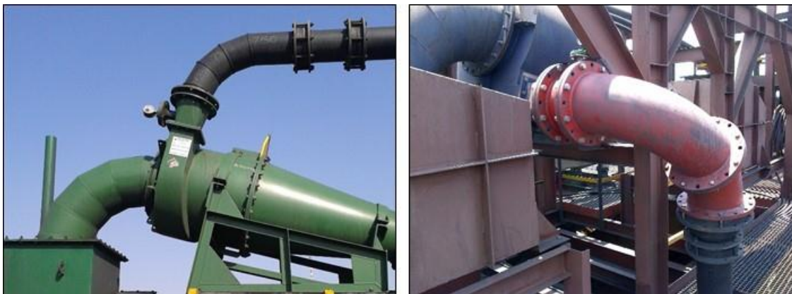
Figure 12: Non-optimal installations of bends prior to cyclones.
