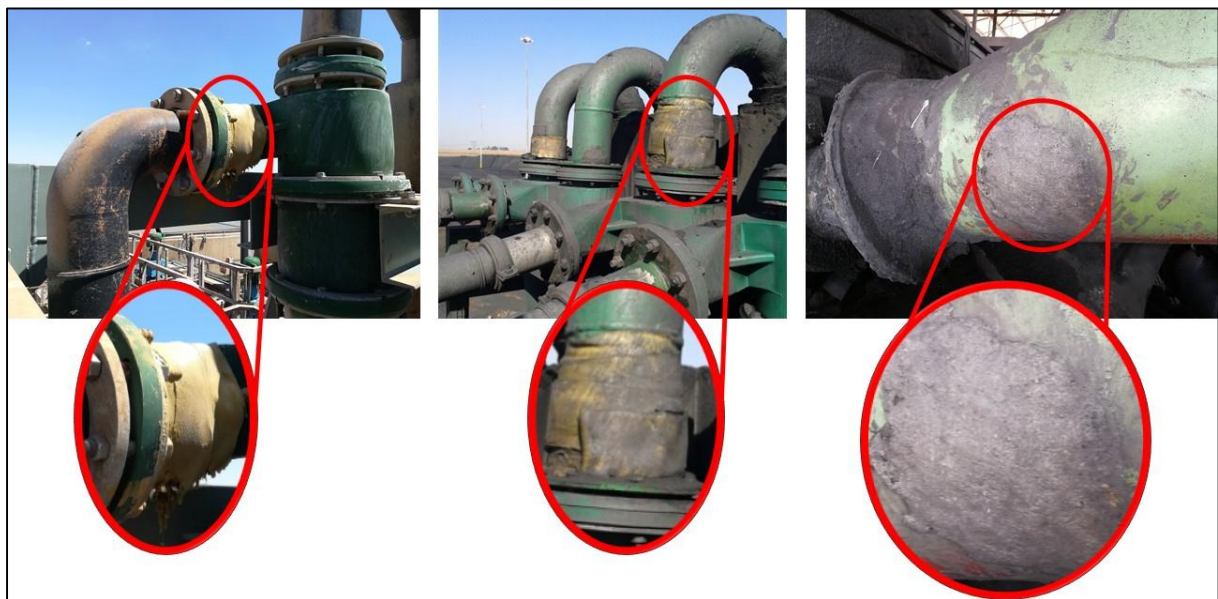
Figure 19: Patched cyclones in operation.
