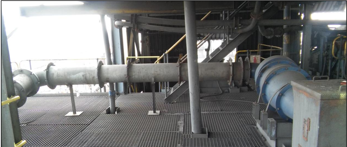
Figure 15: Cyclone installation with horizontal surfaces that is prone to cause blockages.
